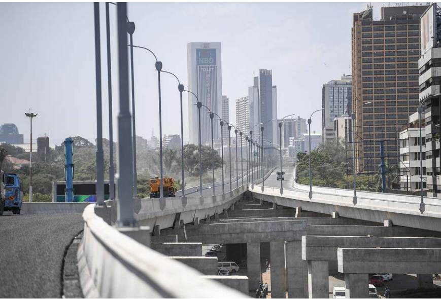
LEFT: A general view of the Nairobi Expressway along Mombasa road in Nairobi.
